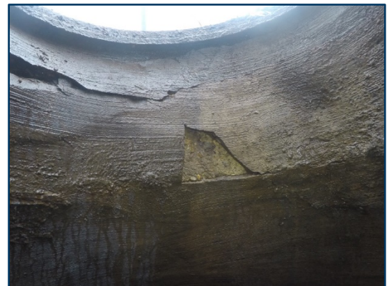
Defective Chimney (BR-03) 50110
