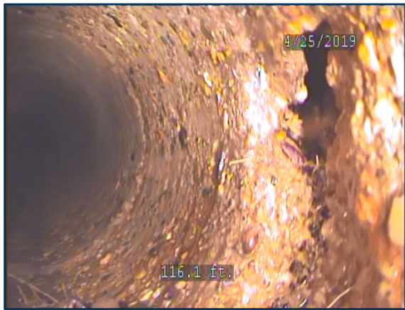
Pipe with hole (BR-03) 50445:50430
